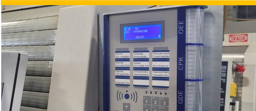
A newly installed data collection terminal
